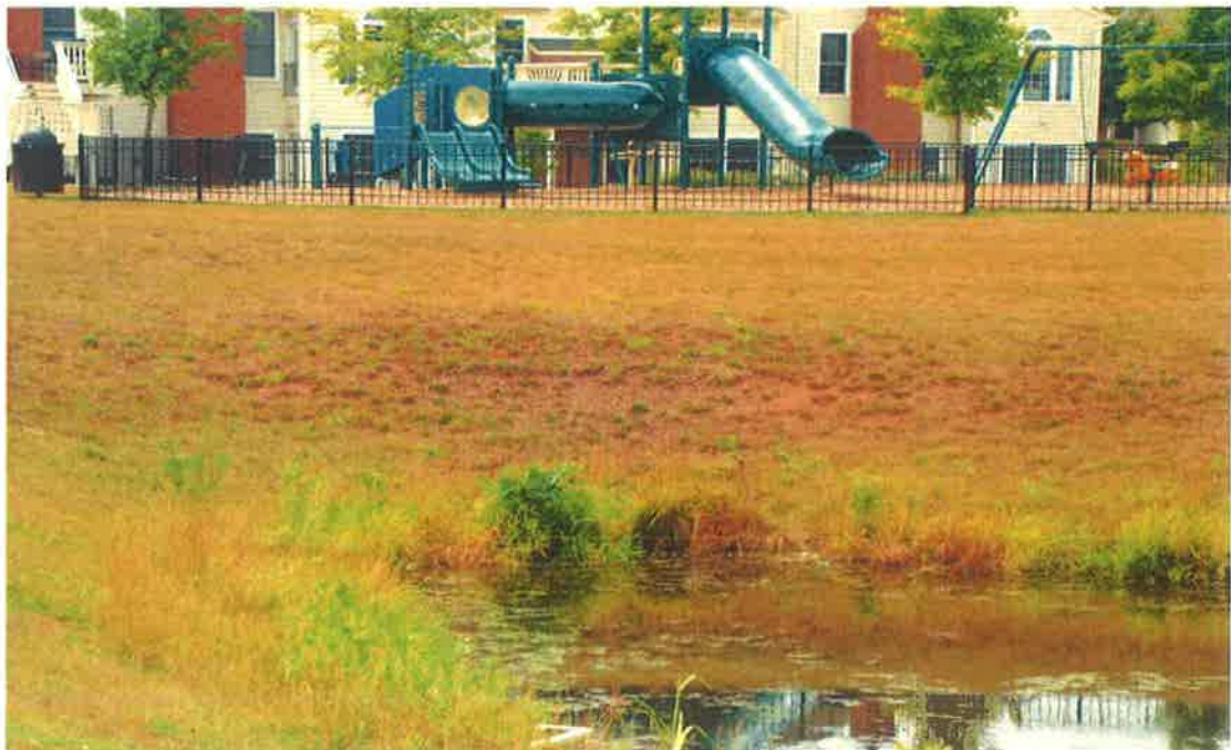
Shore stabilization needed at pond on Arnold Palmer Dr. Reseeding is recommended.
