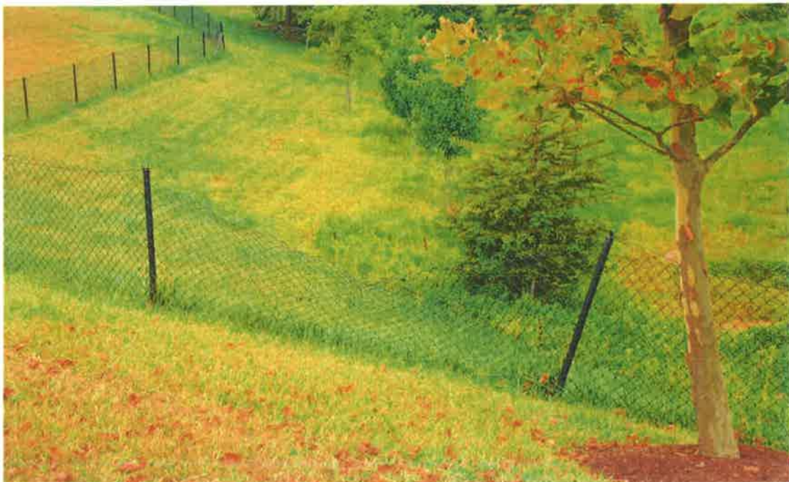
Sagging fence section at SWM pond on Bowers Hill Dr. installation of a top rail would help prevent this from happening elsewhere.
