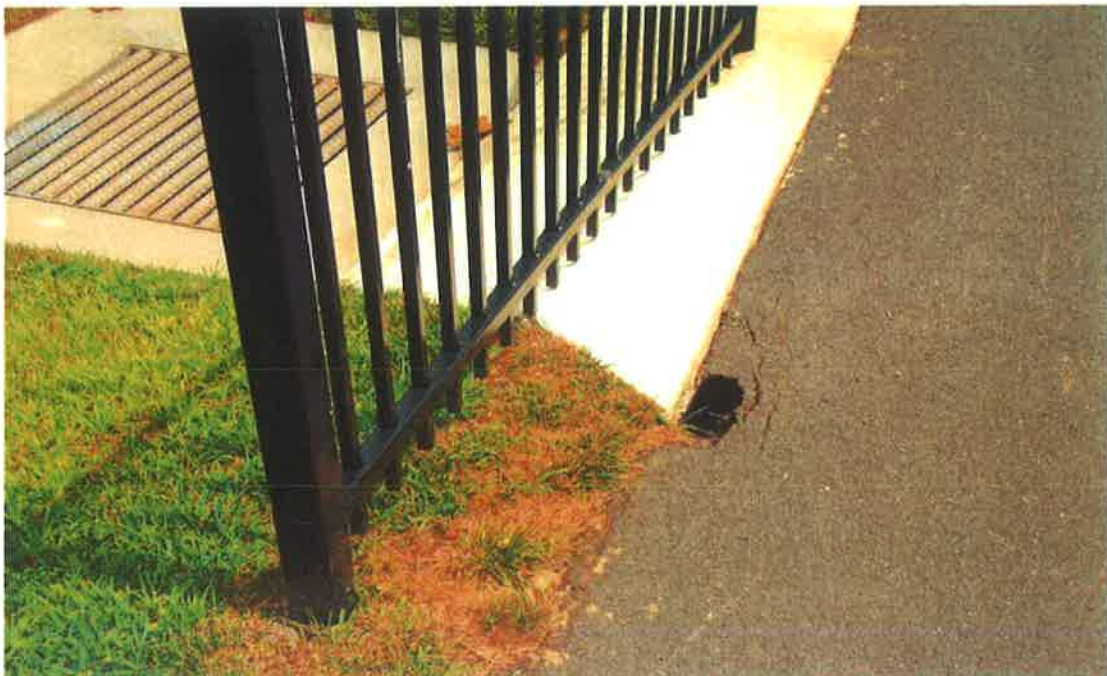
A sink hole exists in the path between the pool and the tot lot at Ryder Cup recreation center.
