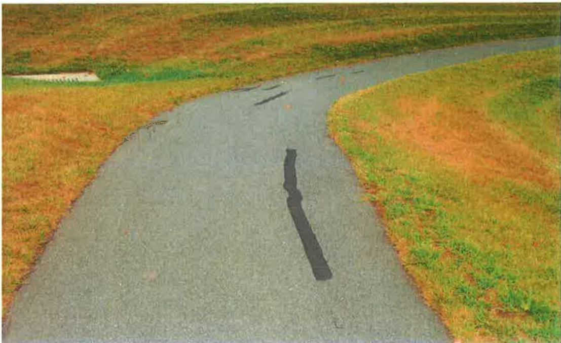
Previously filled cracks in an asphalt path.
