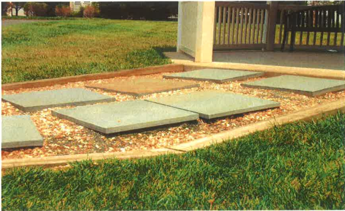
Erosion at walkway to Waverly Park Gazebo.
