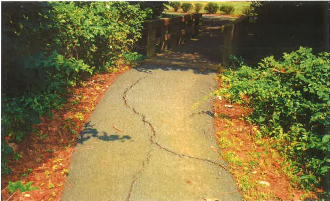
A large crack in the asphalt path off of Walking Stick that should be filled.
