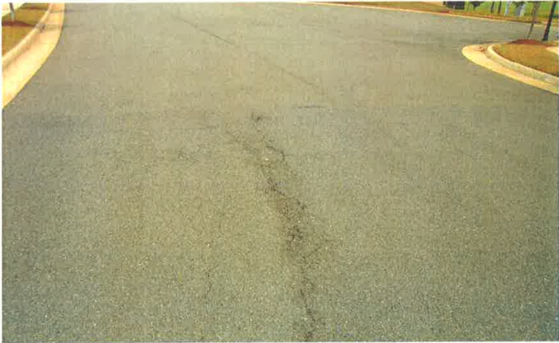
Pavement cracks in isolated areas should be filled to prevent damage from freeze/thaw cycles.
