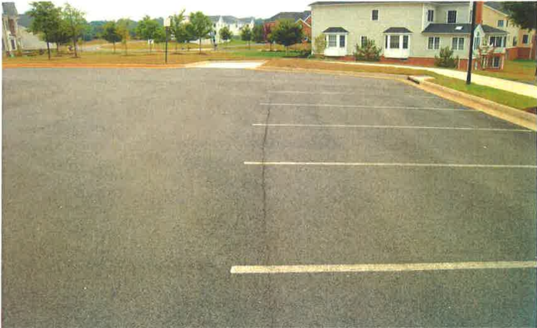
Pavement crack in the recreation center parking lot.
