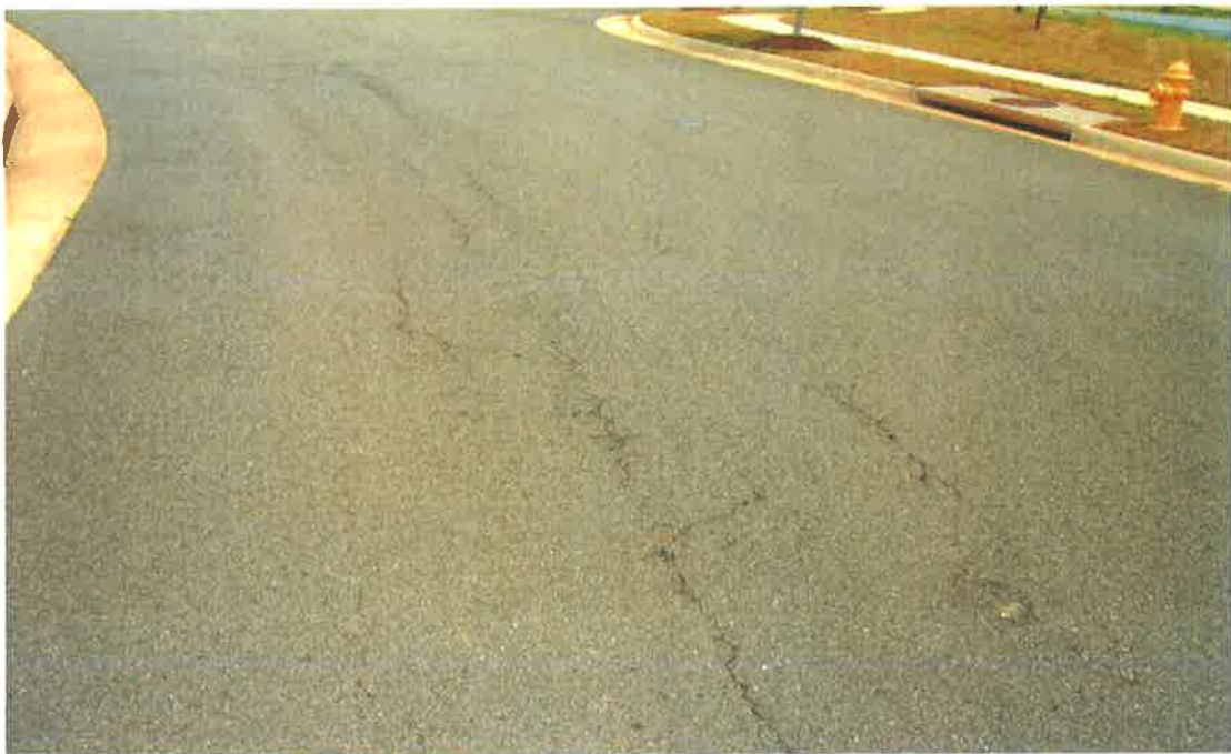
More isolated pavement cracks that need to be filled.
